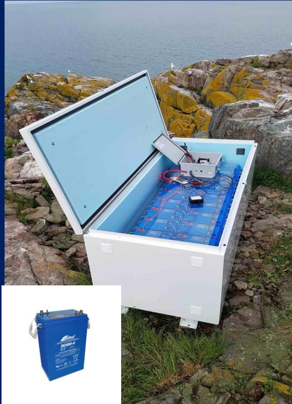
Batteries (Qty: 18) Arranged in pairs to make a 12V system
